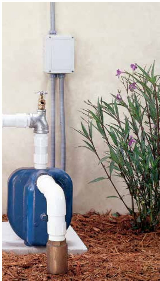
pump start relays
